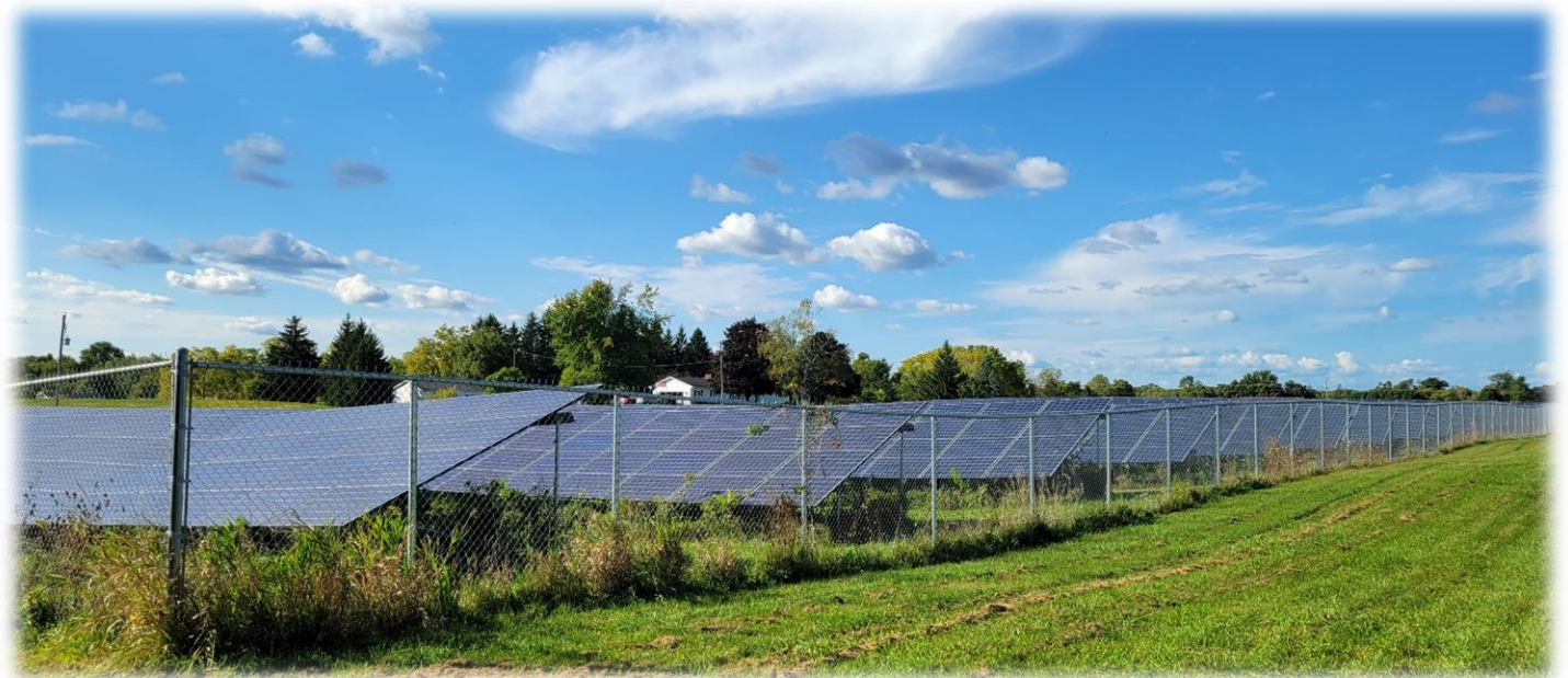
Onsted Schools Solar Project
