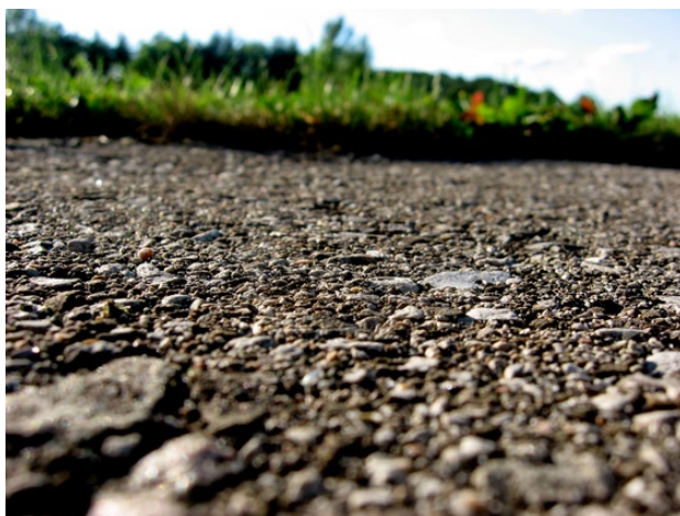
Figure 10-1 Weathered Asphalt Road
