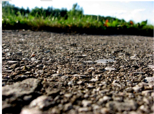
Figure 10-1 Weathered Asphalt Road
