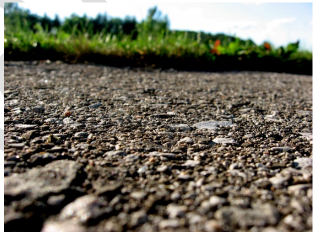
Figure 10-1 Weathered Asphalt Road
