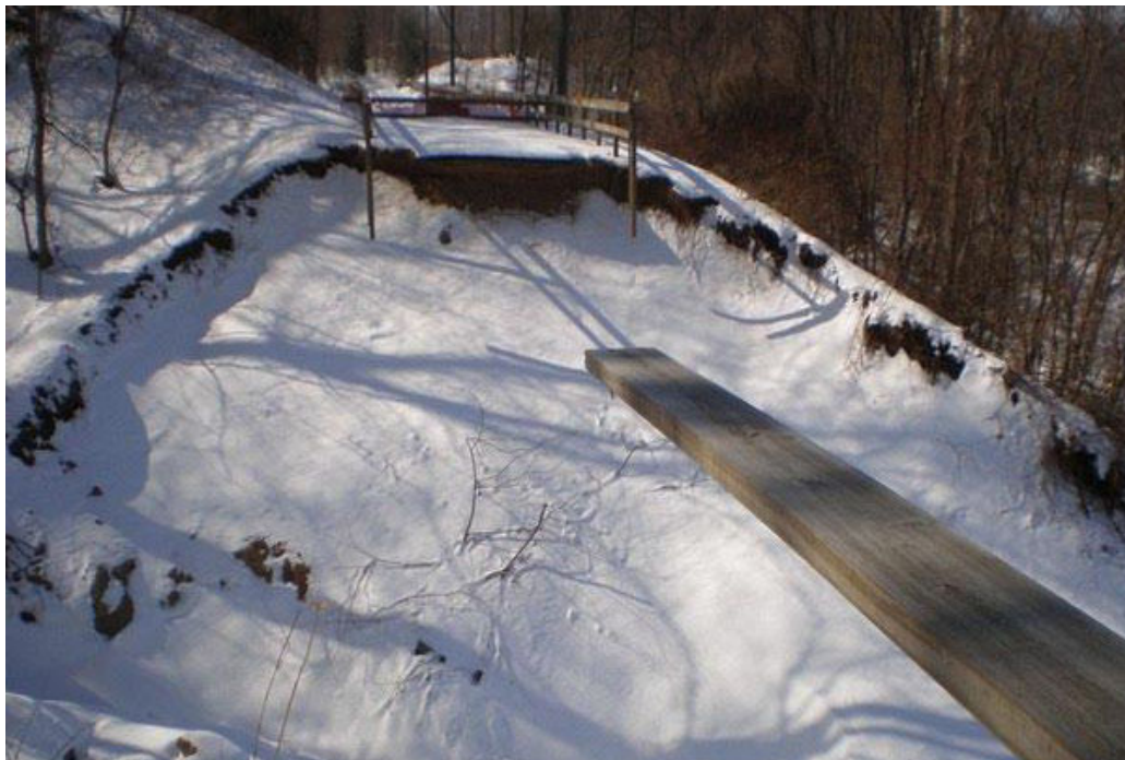
Culvert failure, Manhan Rail Trails, MA.
