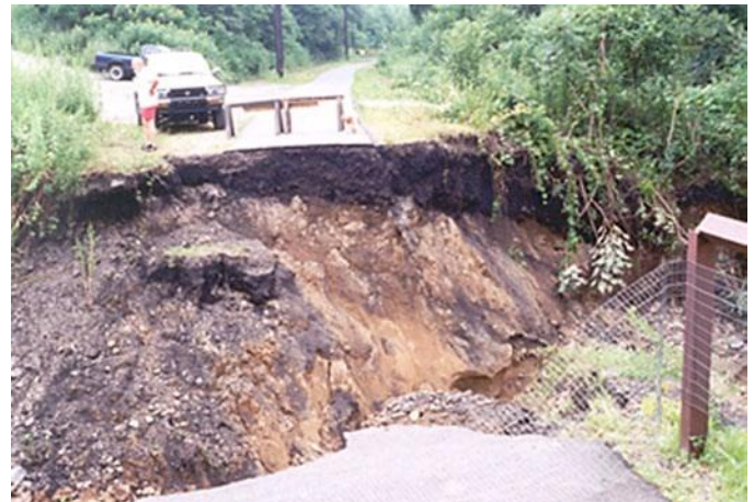
Culvert failure, Allegheny River Trail, PA.
