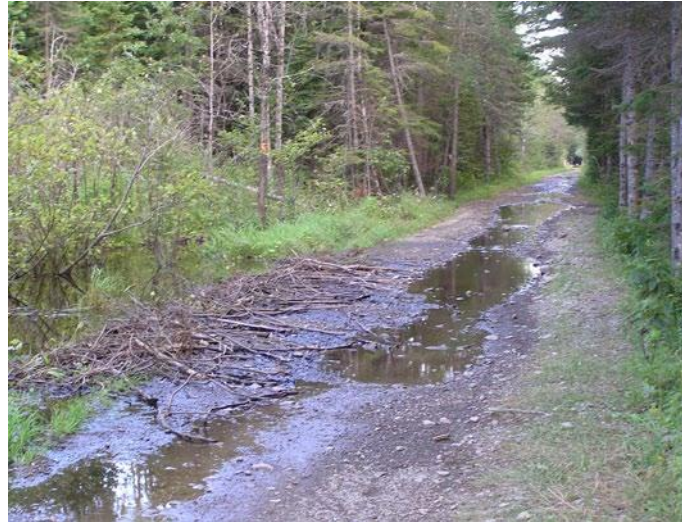
Beaver caused erosion damage, Ashuelot Rail-Trail, NH.
