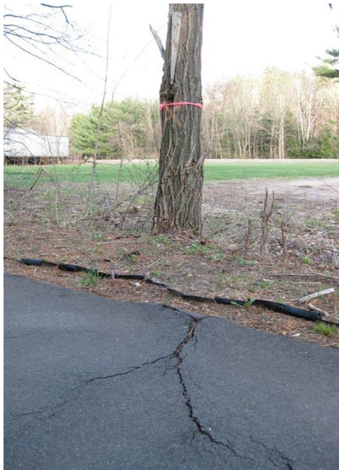
Tree root damage Manhan Rail Trail, MA.
