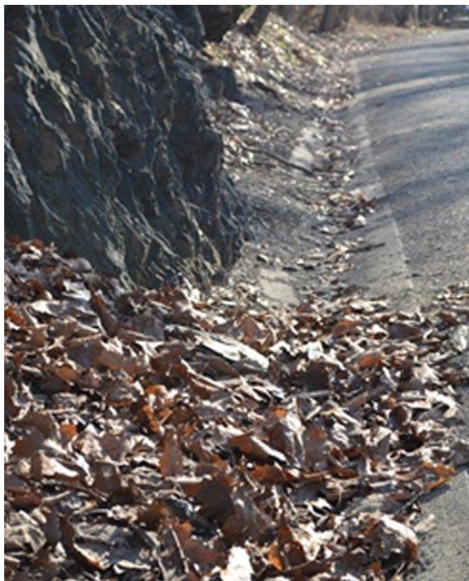
Drainage swale in need of cleaning.
