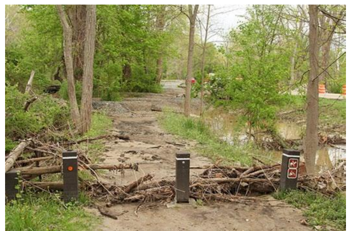
Erosion damage to stone dust trail.
